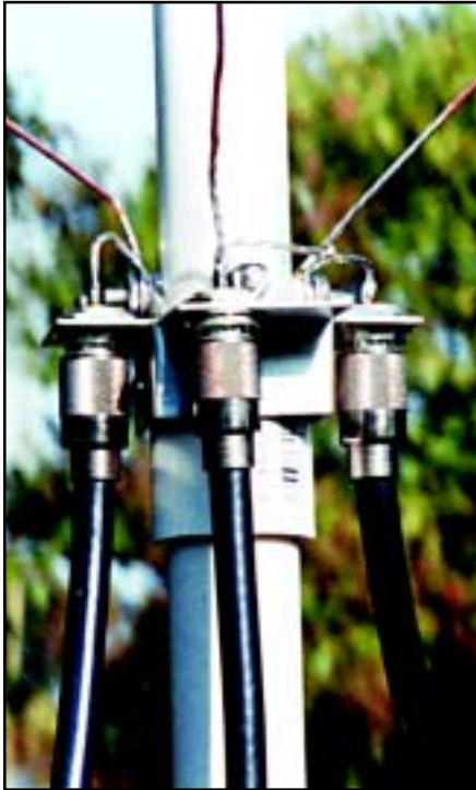
A close-up view of the base and connector assemblies. The photo preceded the final waterproofing of all exposed connections.
